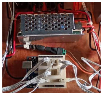
Gambar 1 Pengujian Power Supply
