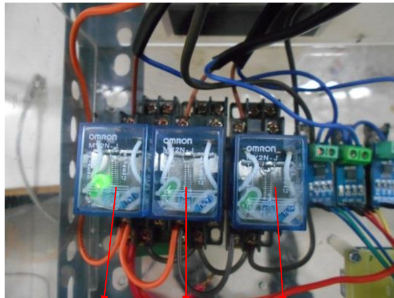
Pompa 1 ON Pompa 2 OFF Pompa 3 OFF
