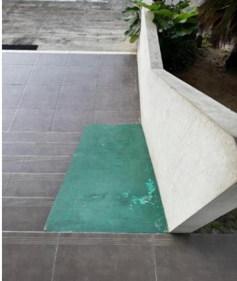
Figure 3. Ramp Not Meeting Standards
