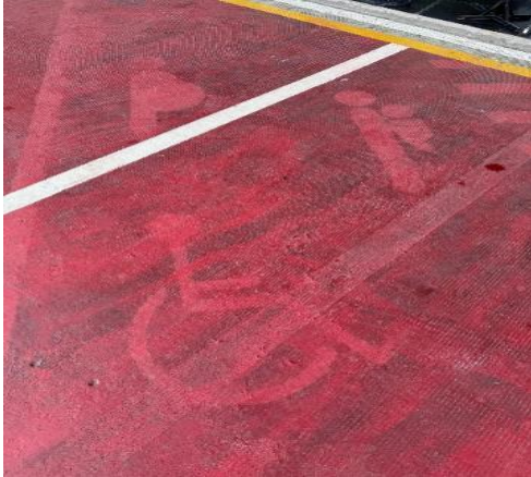
Figure 7. Special Marking Covered by Red Paint
