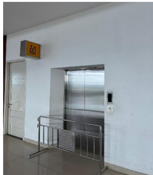
Figure 2. Elevator in the Arrival Area That Cannot Be Used
