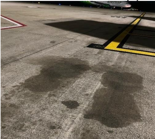
Figure 7. residual fuel/oil spills from a GSE
