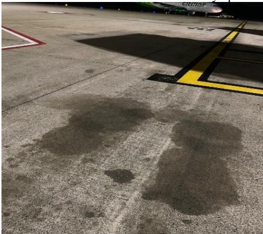
Figure 7. residual fuel/oil spills from a GSE
