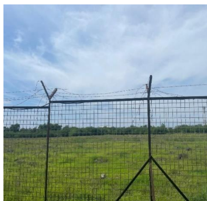
Figure 2. Condition of the Barbed Wire on the Perimeter Fence at El Tari International Airport in Kupang Source: Researcher's Analysis (2024)
