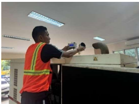
Figure 13 Genset 80KVA Measurement
