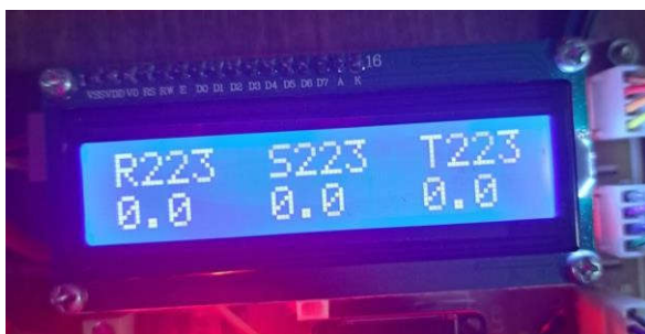
Figure 4 Measurement of Voltage using PZEM-004T
