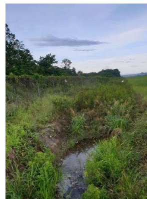
Figure 3.3 Perimeter fence covered with vines the need for maintenance on the perimeter fence and the surrounding area including drainage so that creepers do not grow and make it difficult for officers to carry out checks.
