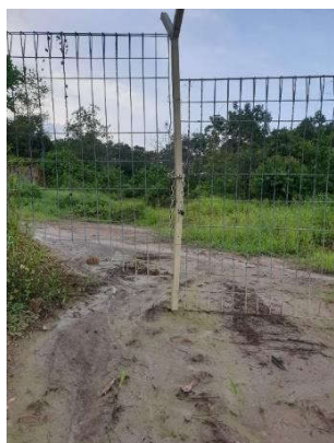
Figure 3.1 There is a gap under the perimeter fence.
