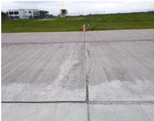
Gambar 6 Kerusakan corner spalling (Sumber: PT. Angkasa Pura II)
