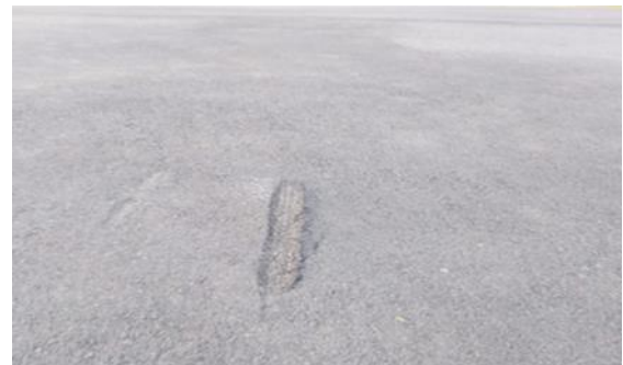
Gambar 2 Kerusakan corrugation and shoving (Sumber: PT. Angkasa Pura II)
