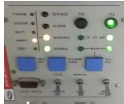
Gambar 4. Tampilan Front Panel Marker Beacon Normarc NM7050 di Bandara Juanda, Sidoarjo.
