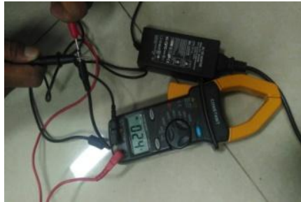
Gambar 8. Pengujian Power Supply
