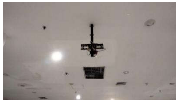
Figure 3. FIDS is not installed yet
