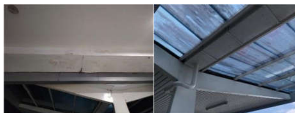
Figure 4. Ceiling on the Leaking Hallway
